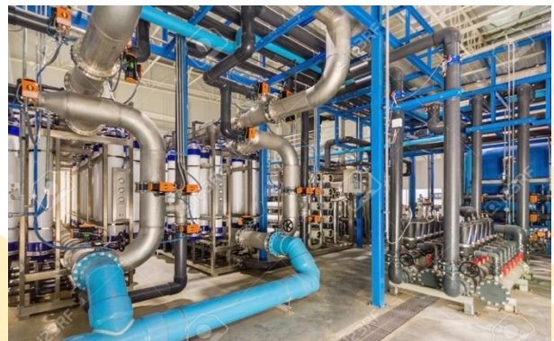
Image 9: Reverse Osmosis Plant. Example.
