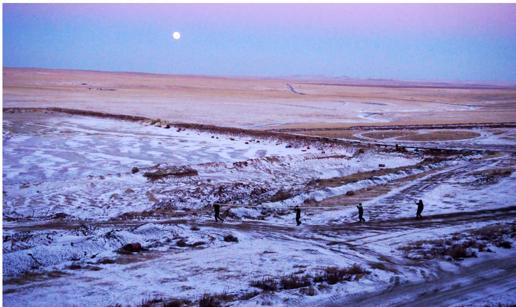
Four workers carry an insulated water pipe across the snow-covered grounds of the mine.
