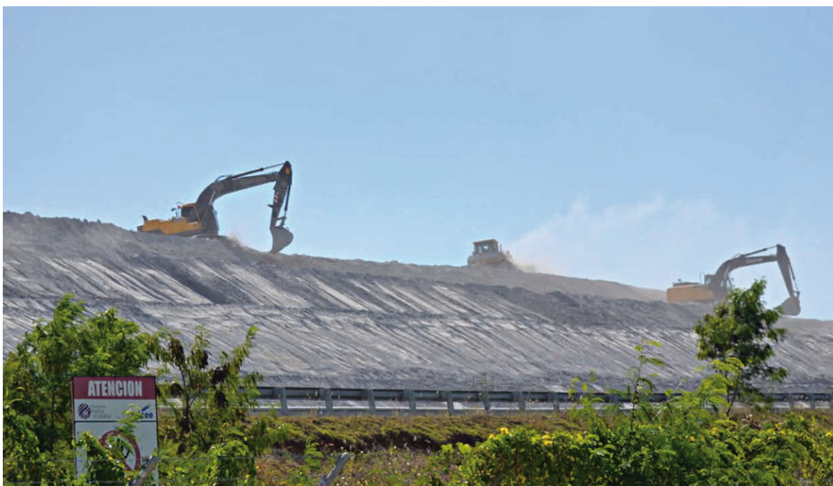
Mountains of toxic ash from the Punta Catalina Thermoelectric Power Plant. Batey San José, Peravia province. April 12, 2021 © CLNCC
