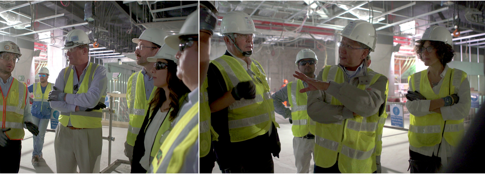
Site visit of the QDVC Underground Pearl Station of the Lusail Light Railway Transit System Project site.
