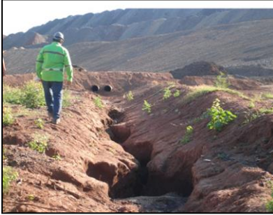
Initial status of channel.
